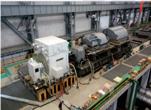
50MW Motor Test Bed
