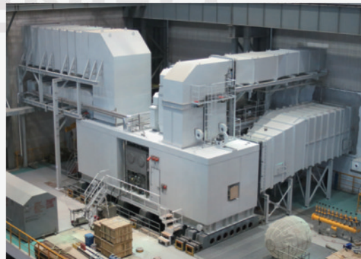
30MW Gas Turbine Test Bed
